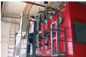
Steam dome of an 840 kW boiler
