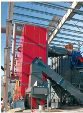
8000kW Sunnyside Greenhouses Ltd
